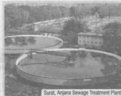
Surat, Anjana Sewage Treatment Plant
